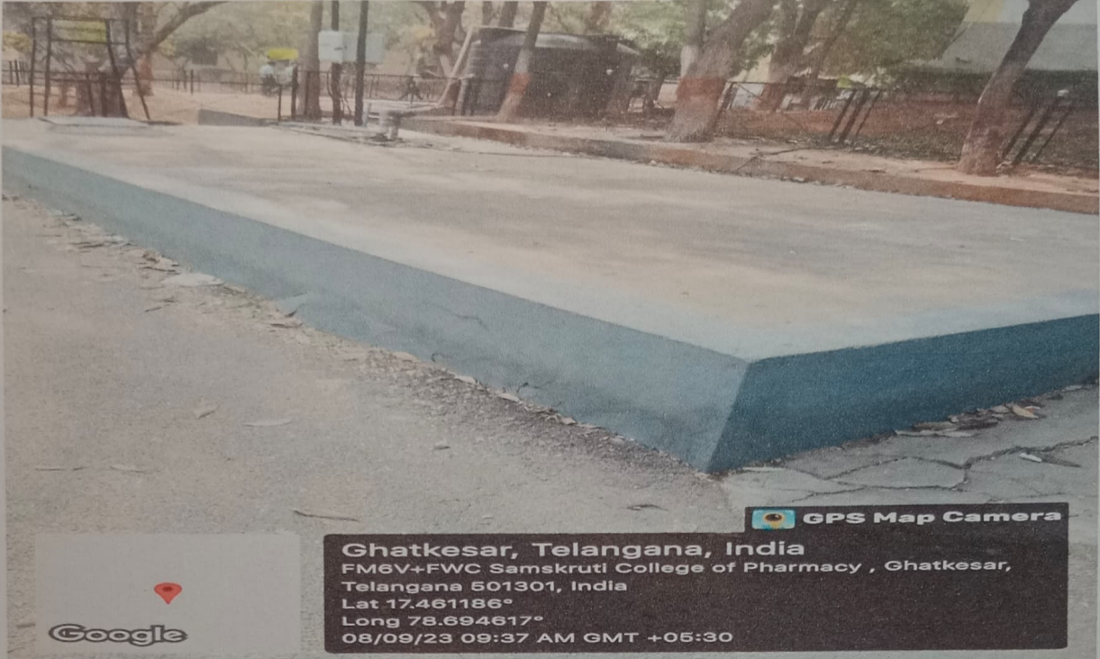
Common Water tank
